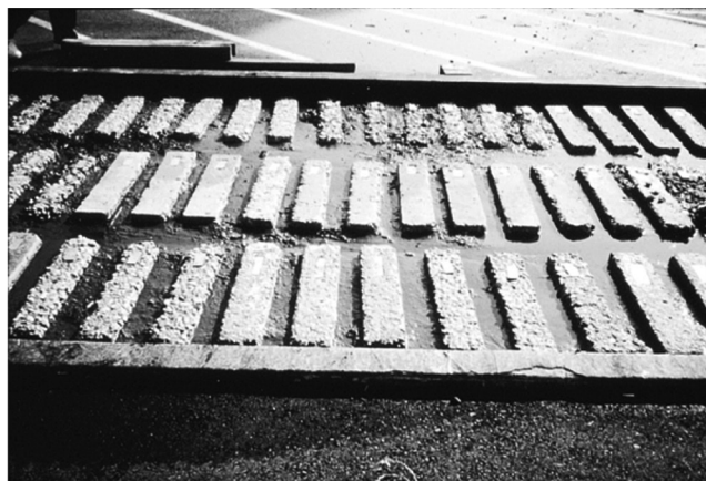
Fig. 3.3—Concrete beams after 7 years in sulfate-rich soil in Sacramento, CA, test facility.
