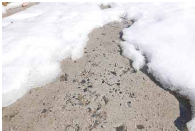
Typical scaling problems that were happening in the Northeast United States due to harsh winters
