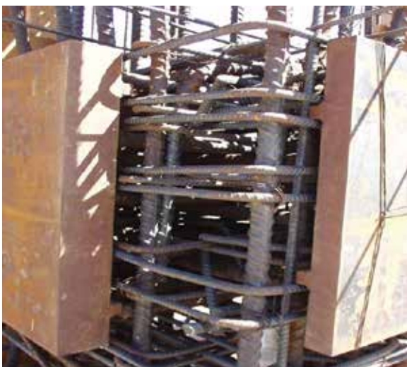
Fig. 3: Reinforcing bars must clear embed plates and studs by the clearance provided in Section 2.3.1 of ACI 117, and the SER must provide details showing how the clearance is to be maintained. This is particularly critical when the embeds have very thick plates
