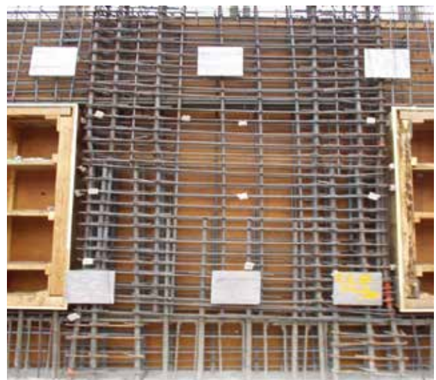
Fig. 5: A reinforced concrete wall with embeds and penetrations, shown prior to closure of the formwork. The embeds adjacent to the wall penetrations interfere with the vertical bars in the wall
