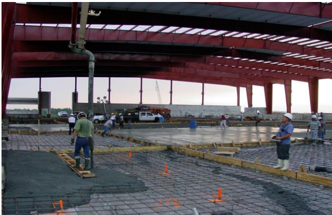
Fig. 5 Waste Transfer Station durable floors
