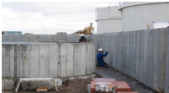
Fig. 4 Chemical Storage & Containment Areas
