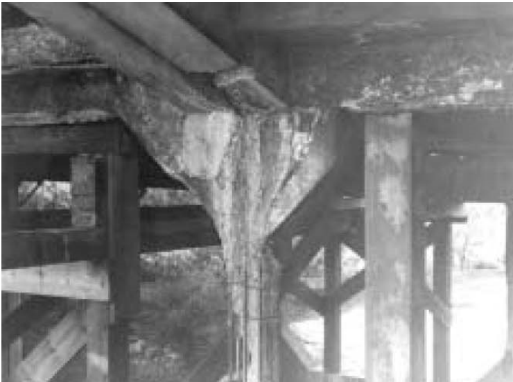
West 6th Street Viaduct in Erie, Pennsylvania prior to repair
