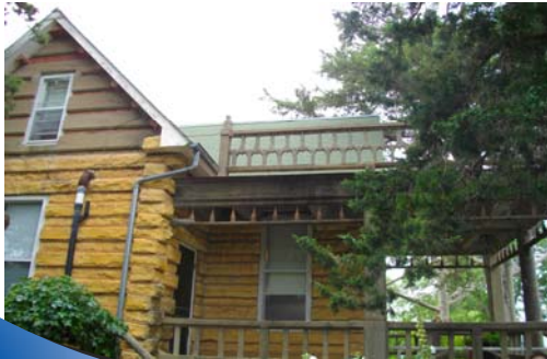
The 3rd story (the gables), floors, baseboards & the window stools were all made of concrete.
