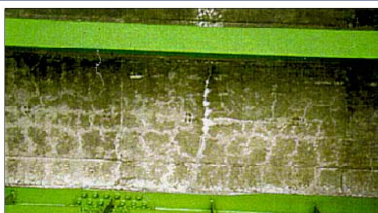
Photo 1: Evidence of cracking in concrete on underside of the deck slab
