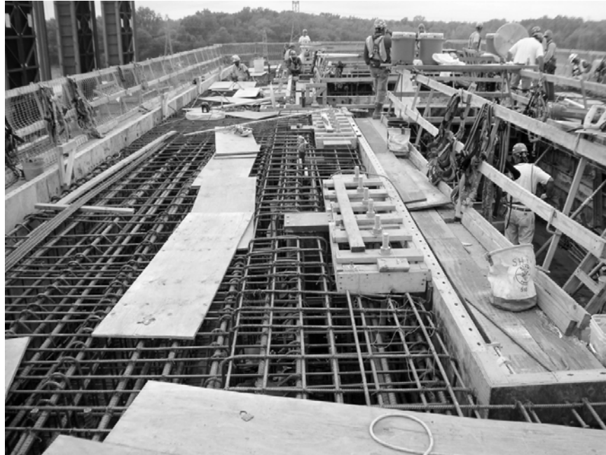
Figure 1 Overview of beams showing reinforcement congestion.
