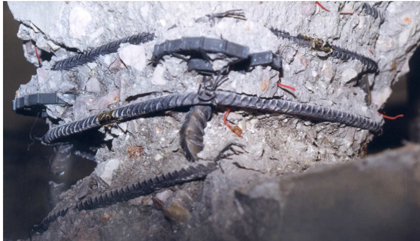
Typical failure of a column's upper part.
