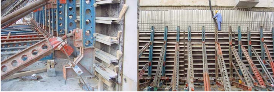
Fig.8 - With SCC at high casting rates, the formwork should be strengthened especially at the bottom (Courtesy of M Sonebi)
