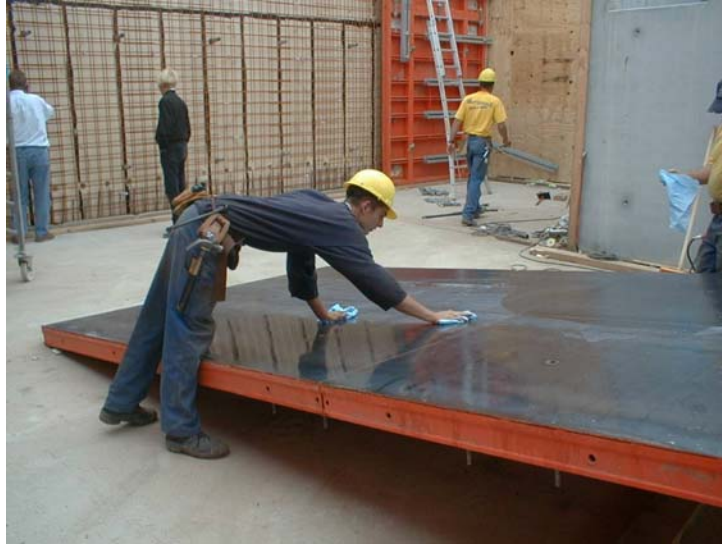
Fig 10 - Properly prepared formwork is important for high surface quality (Courtesy of G. De Schutter)
