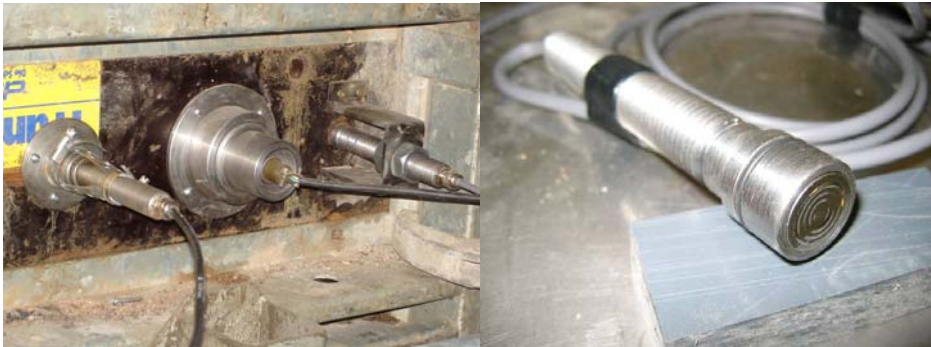
Fig 7 - Formwork pressure could be monitored using (small) pressure transducers, flush with the form panels (Courtesy of V. Dieryck)
