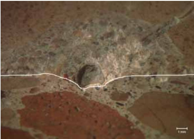
Fig. 1: Popout due to alkali-silica reaction (photographed at an angle). The white line delineates the boundary between the top surface (above line) and the polished surface perpendicular to it (below line). The offending shale particle can be observed in the base of the popout
