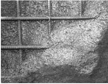
Fig. 8.12—Proper encapsulation of reinforcing steel. Good compaction and proper velocity. Note glossy appearance, bar deformation, and even build-out of shotcrete.
