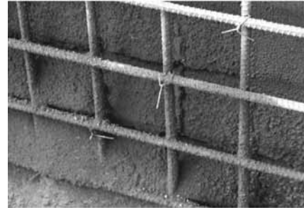
Fig. 8.14—Example of poor encapsulation. Material is too dry and shadows have formed behind bars. Also note obvious valleys in shotcrete material.
