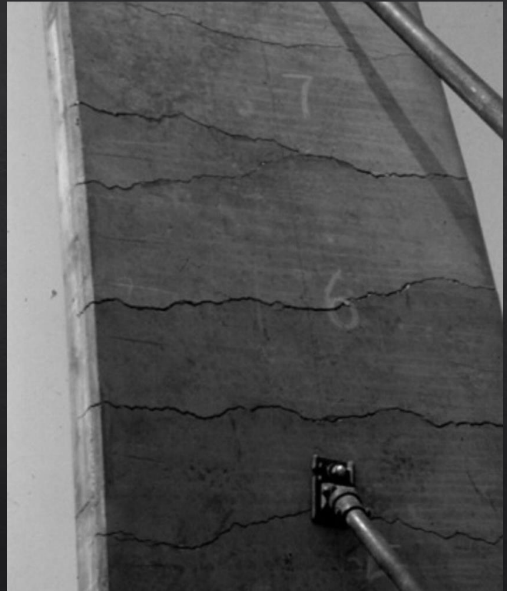
TEST PANEL CRACKING
