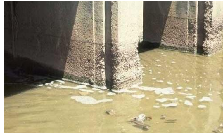
Concrete exposed to sulfate rich water
