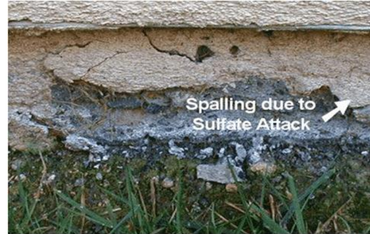
Concrete exposed to sulfate rich soil
