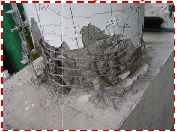
Typical plastic hinge in cast-in-place construction after a large earthquake
