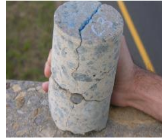
C3 - delamination at 3.5 inches
