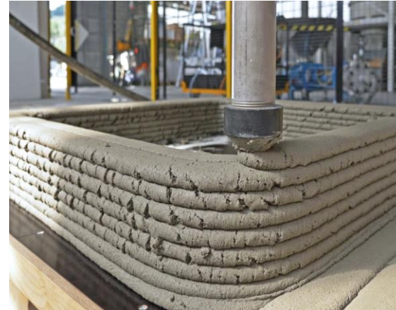
Plastic shrinkage and cracking
