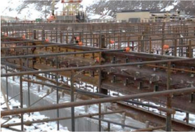
Fig. 8: Steel-panel bulkheads with horizontal corrugations were used as a form between sections
