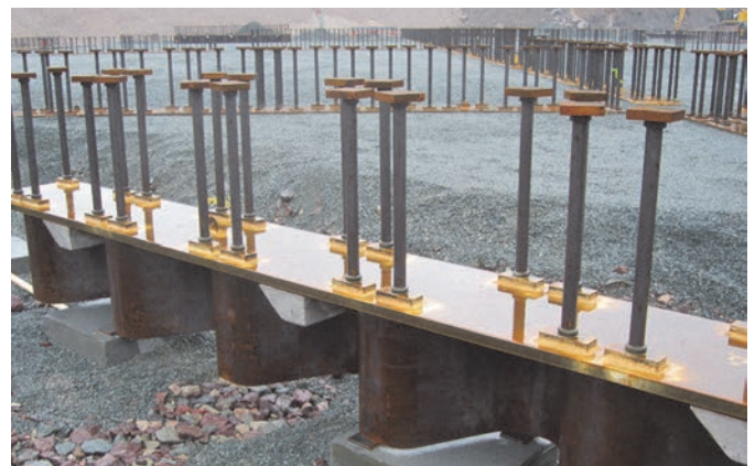
Fig. 6: Steel skirts with T-headed bars were installed below the base slab to increase sliding resistance
