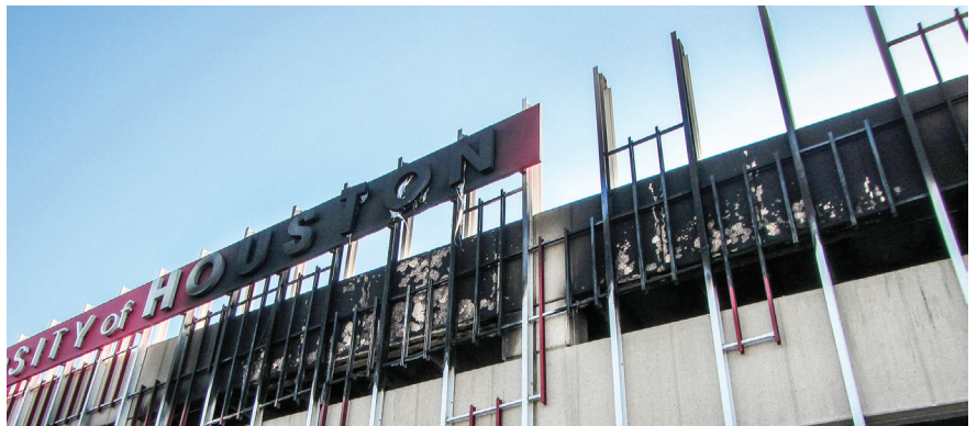
Fig. 3—Fire damage at exterior of garage
