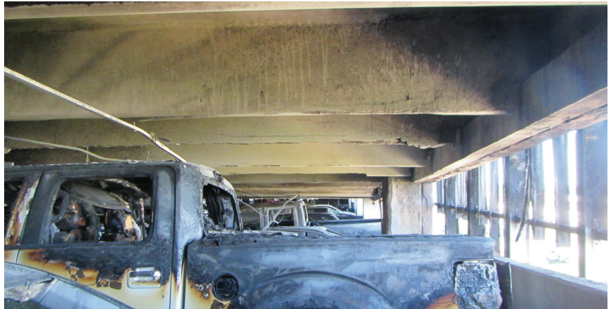
Fig. 2—Fire damage on Level 3 of parking garage
