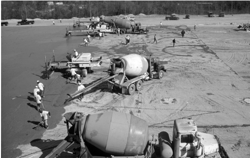
Fig. 1.2—Construction schedules and contractor economics typically require concrete placements of 10,000 to 20,000 ft 2 (900 to 1800 m 2 ) or from 30,000 to 50,000 ft 2 (2800 to 4600 m 2 ) when a laser-guided, wheel-mounted screed is used. This figure shows a 300,000 ft 2 (27,900 m 2 ) placement that was completed within 24 hours.
