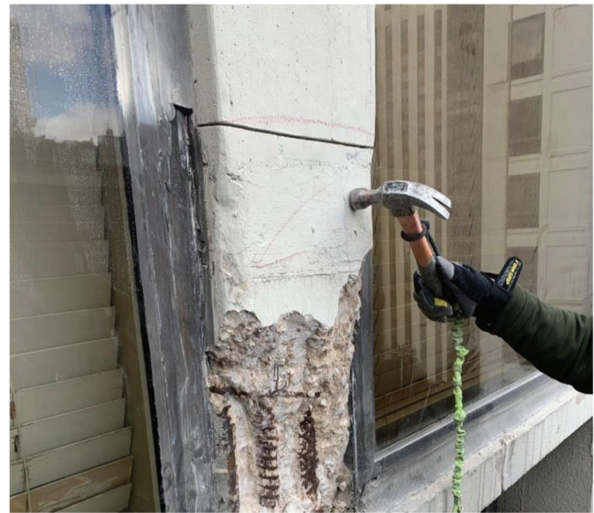
Fig. 1.1—Deteriorated concrete column on building façade.
