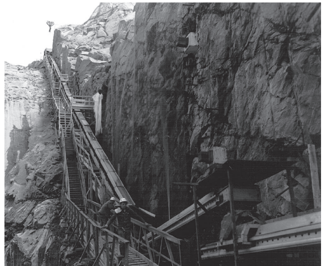
Fig. 4.3b—Feeder belt conveyor 659 ft (200 m) on Dworshak Dam spillway operating down 30-degree slope.
