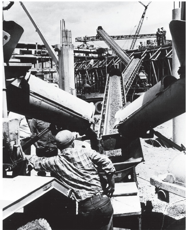
Fig. 5.3—One truck is preparing to discharge while the second truck is discharging.
