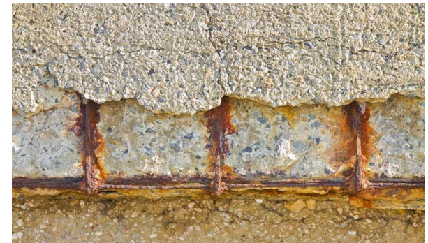
Carbonation induced corrosion
