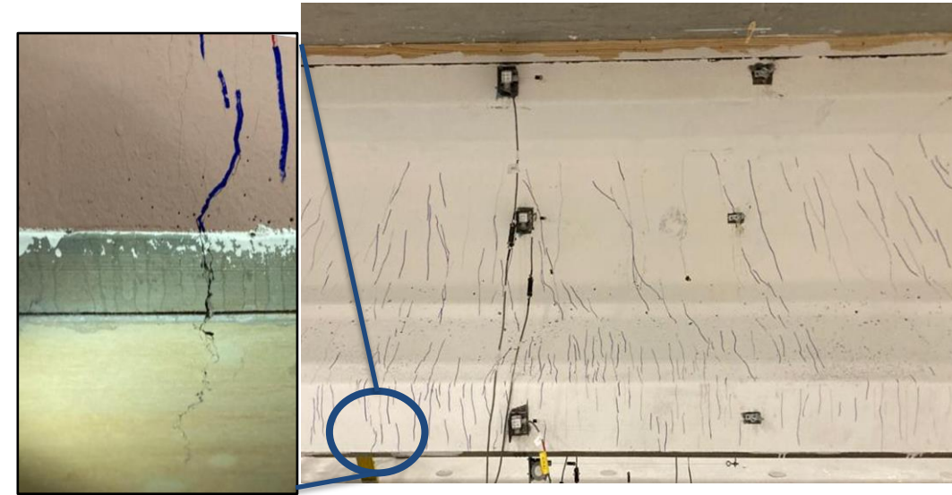
Flexure Cracks Tx34-2
