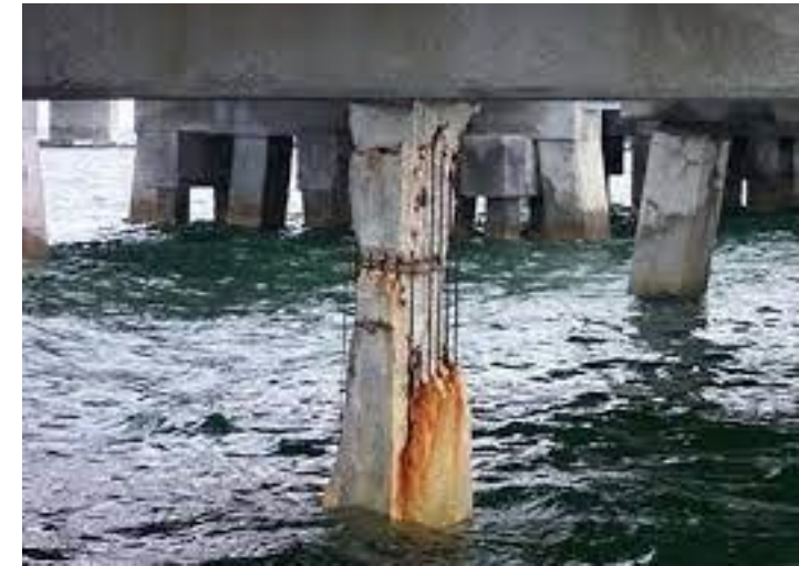
Fig. 1: Deterioration of concrete exposed to seawater
