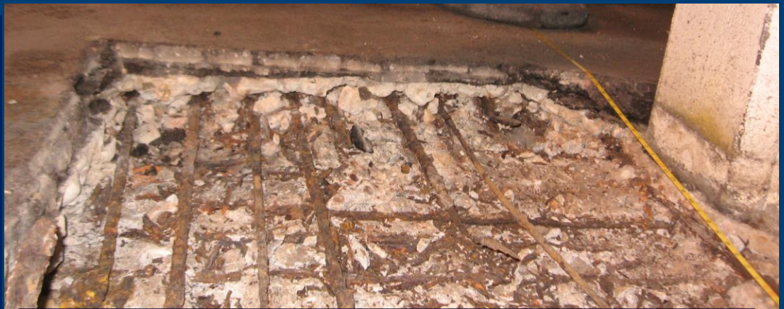
Asphalt overlay conceals concrete spalls at columns
