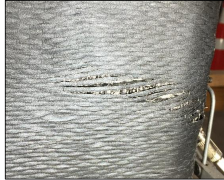
(a) First longitudinal FRP sheet damage - Column 6
