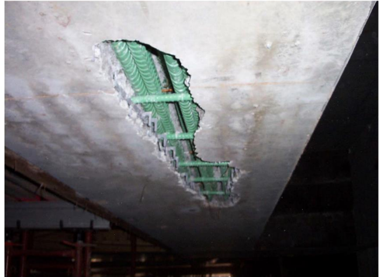
Fig. 16 The end result of using flowing concrete, slump greater than 7\frac{1}{2} in., on a 42 x 68 in. beam that was designed in accordance with ACI Code requirements. The four layers of #10 lap splices in the bottom of the beam prevented concrete flow and consolidation to reach the bottom.
