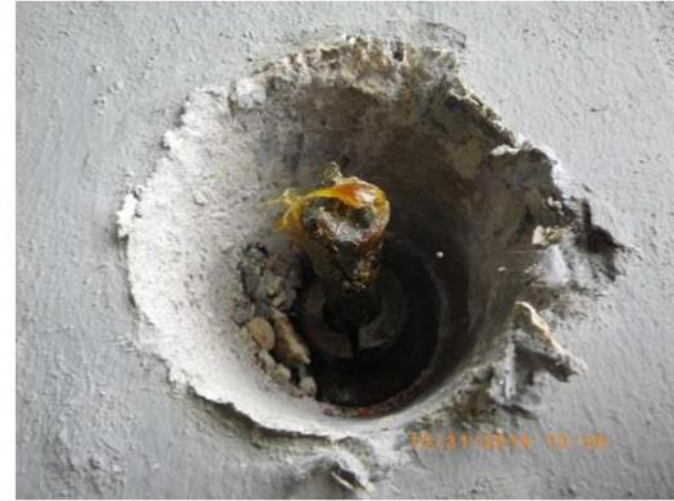
Figure 8. Unstressed strand at location shown in Figure 7 (note wedges were loosely placed grout pocket was removed).
