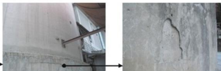
spalling of concrete cover at the silo bottom due to temperature actions from kiln
