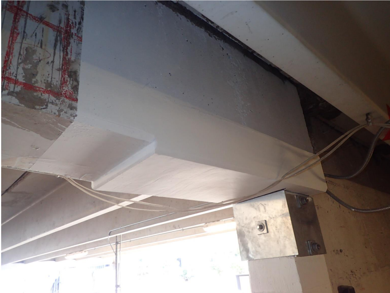
Completed Repair – Drop in beam soffit installed to provide additional cover for reinforcing (not in drive aisle)
