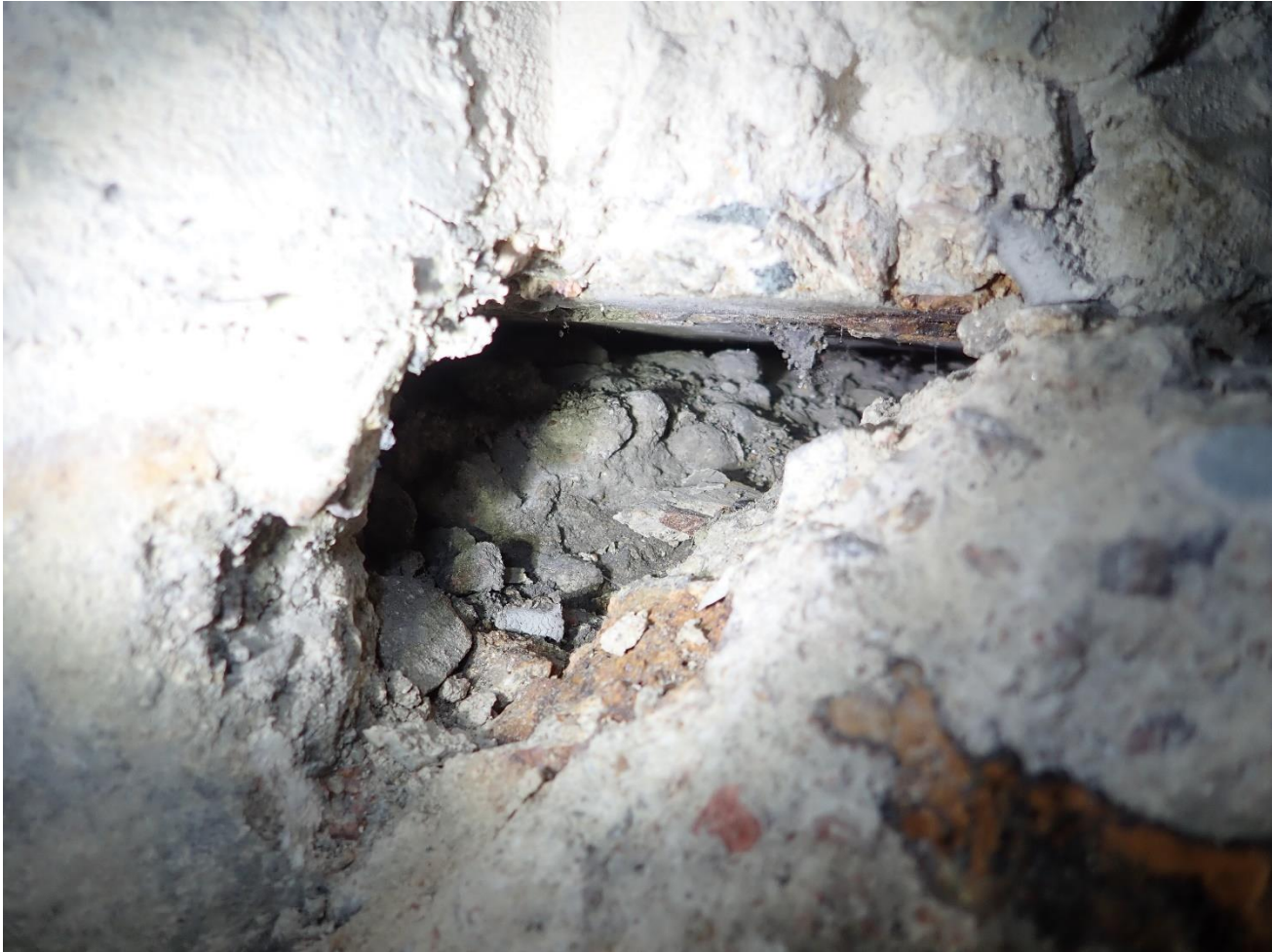
Void below Column
