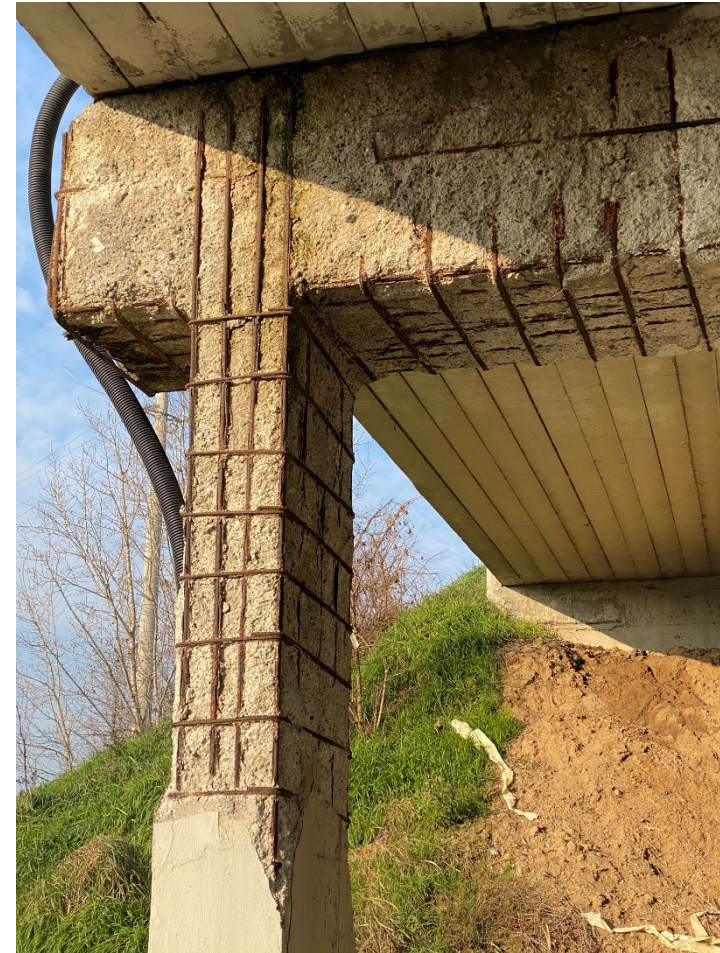
SEVERE REINFORCEMENT CORROSION
