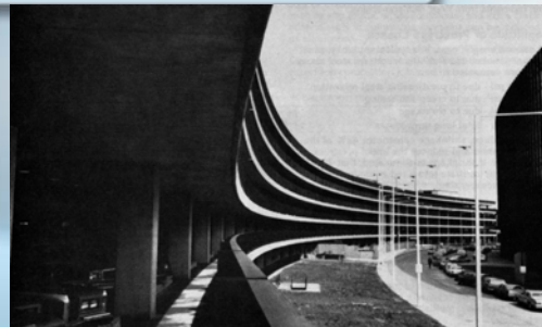
Post-tensioned Type-K cement concrete provides superior durability for Chicago's O'Hare Airport. 9,000 car parking structure constructed in 1973
