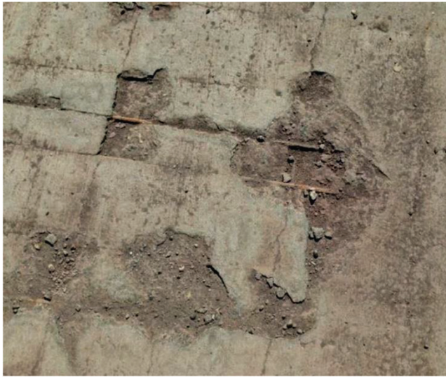
Fig. 3.1.1b—Spalled concrete that will likely need to be addressed prior to installation of a protection system.
