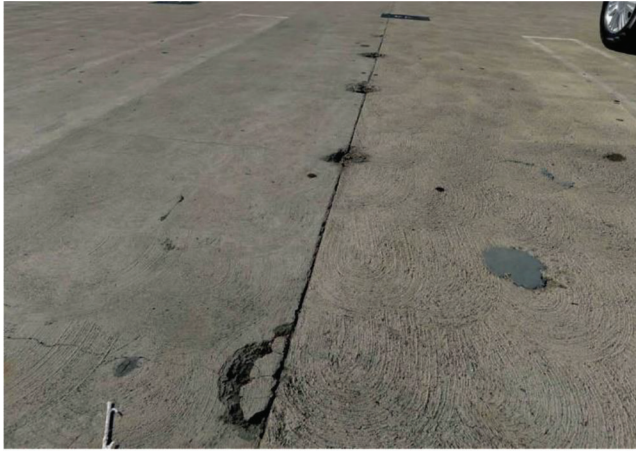
Fig. 3.1.1a—Spalled concrete that will likely need to be addressed prior to installation of a protection system.
