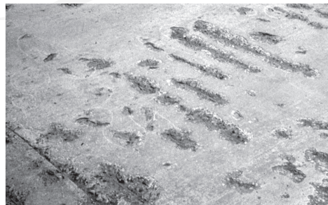
Fig. 4.1e—Shallow cover depth spalling.
