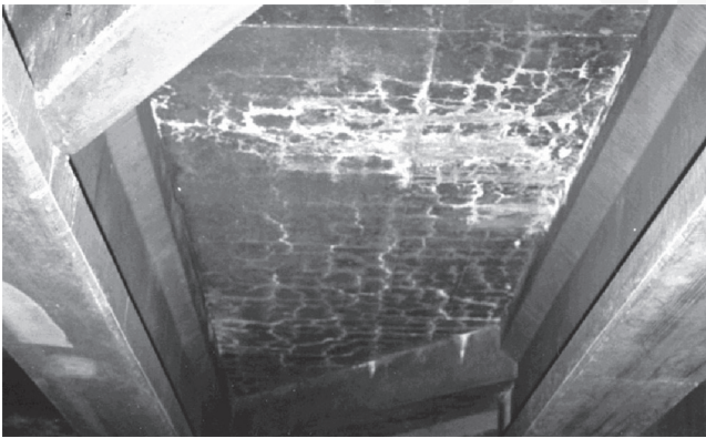
Fig. 4.1b—Map cracking on underside of deck.
