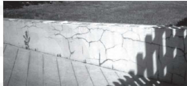
Fig. 4.1d—Map cracking in parapet.
