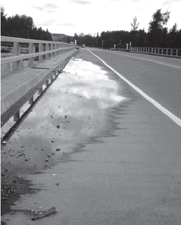
Fig. 4.1a—Water ponding from improper deck drainage.
