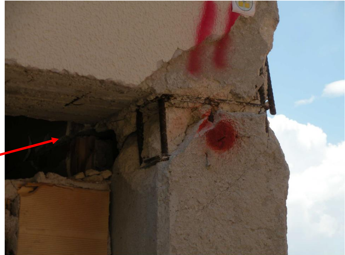
Top column shear failure due to infill-to-structure interaction
