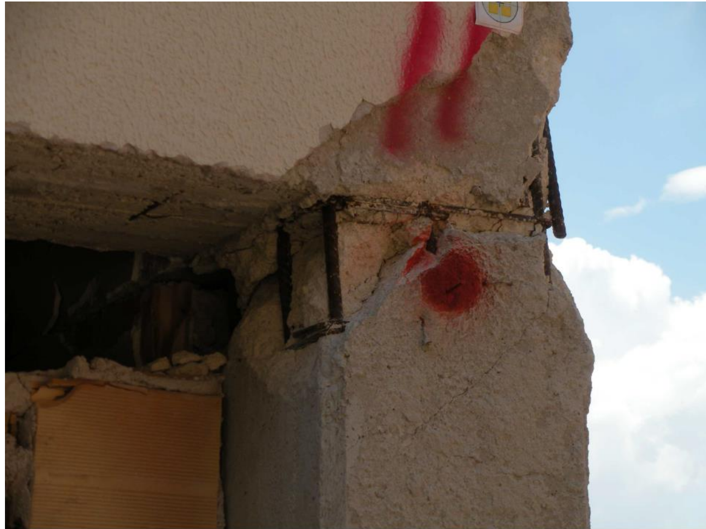
Actual damage detected on the building
