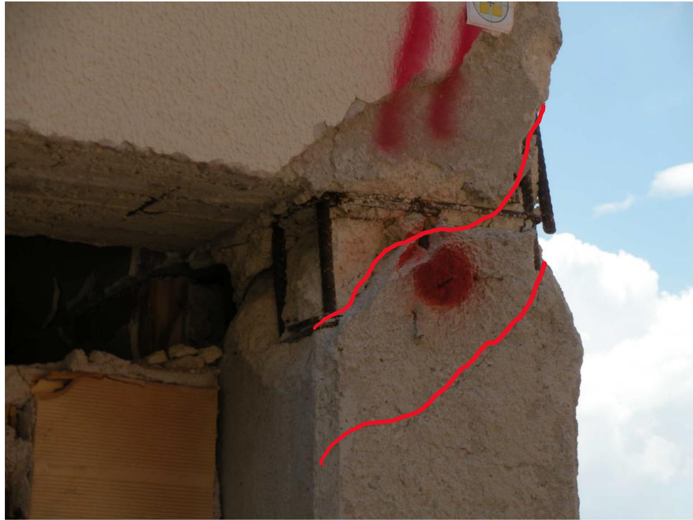
Actual damage detected on the building
