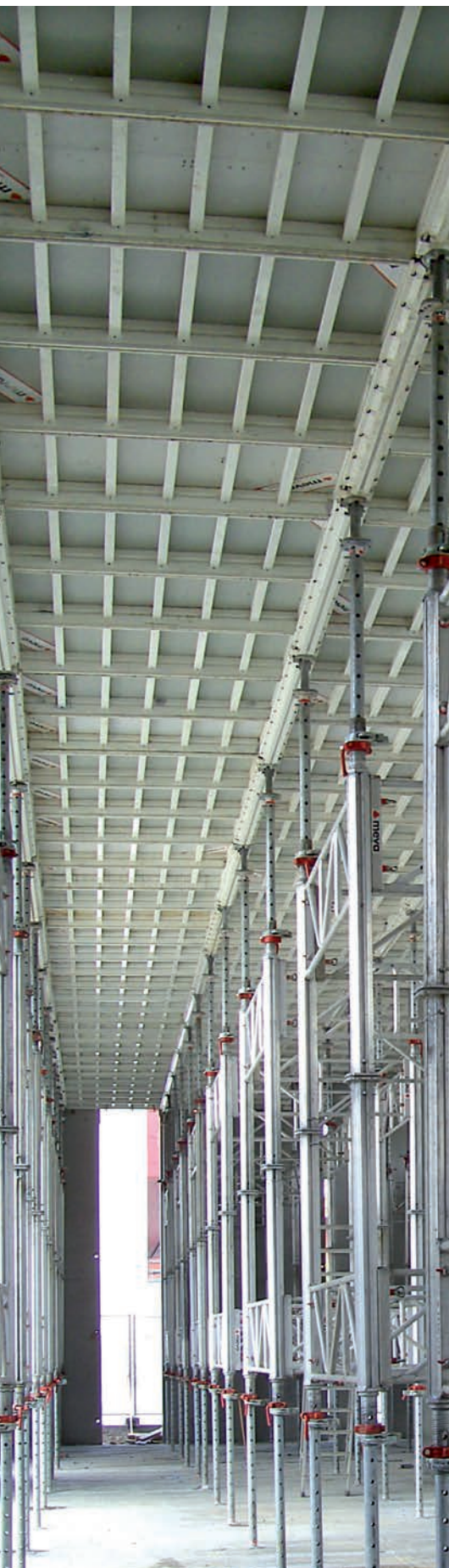
Fig. 1.1: Manufactured metal formwork system for concrete floor slab construction (Photo courtesy MEVA Formwork Systems)
