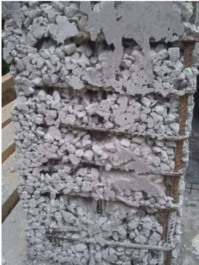
Aggregate Segregation of SCC
