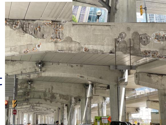
Corrosion in RC Bridge Piers and Pier Caps at Lakeshore BLVD. Crossing Yonge St. of Toronto, ON in July 2023
