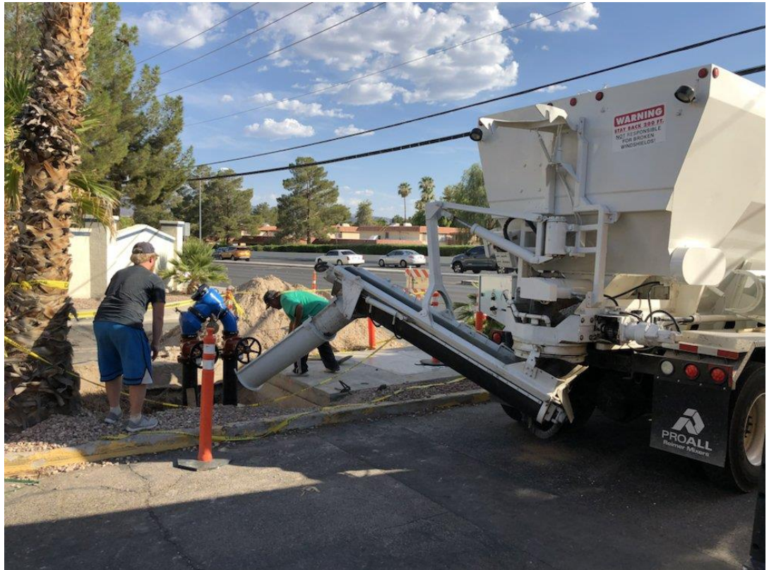
Las Vegas Mobile Mix truck pouring out ready mix concrete for utility works in Henderson, Nevada, 2018
