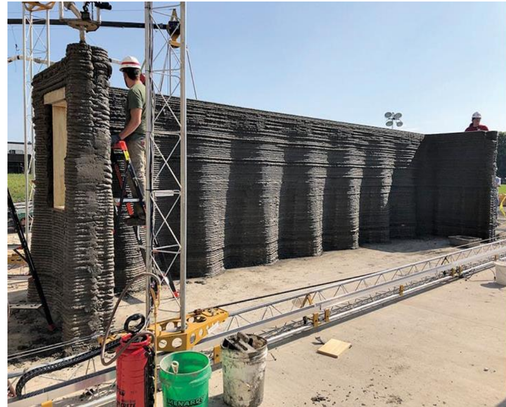
USACE: 3D printing of 9.5-ft-tall reinforced concrete walls for a 32-ft x 16-ft barracks
