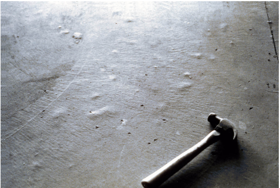
Fig. 0.2—Example of concrete surface blistering (photo courtesy of Portland Cement Association (PCA))
