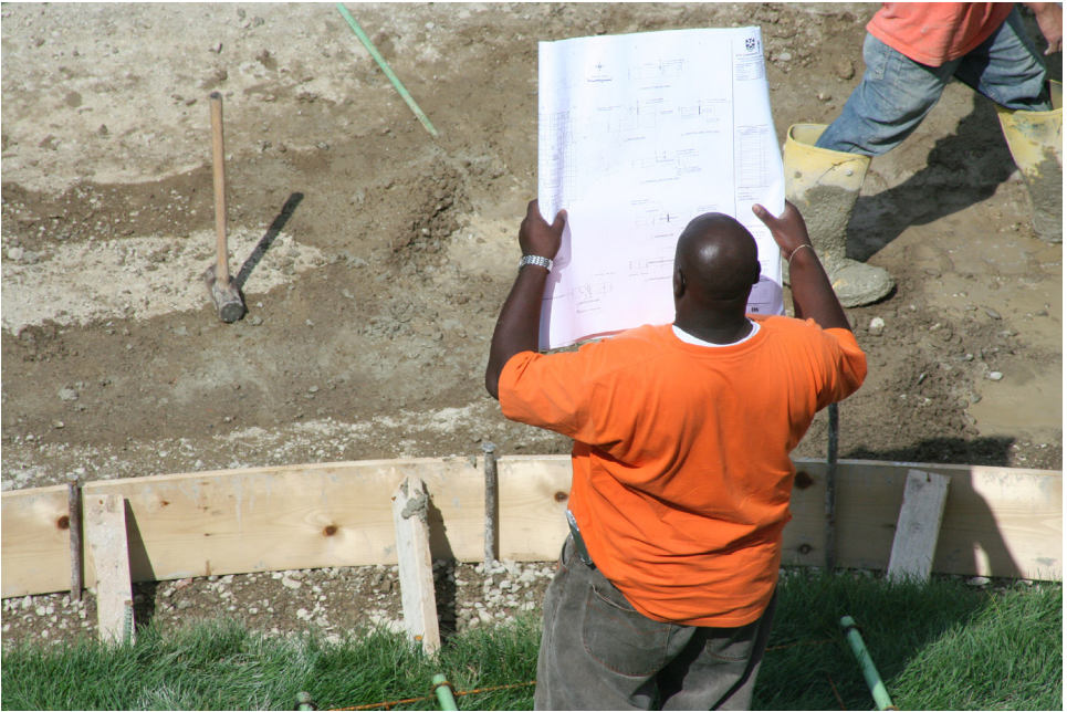
Fig. 0.1—Project plans and specifications should be followed. Practices described in this book are not a replacement for project plans
