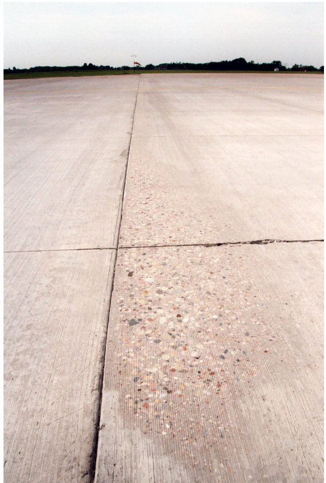
Fig. 0.5—Scaling removes the top layer of paste from the concrete (photo courtesy of PCA)
